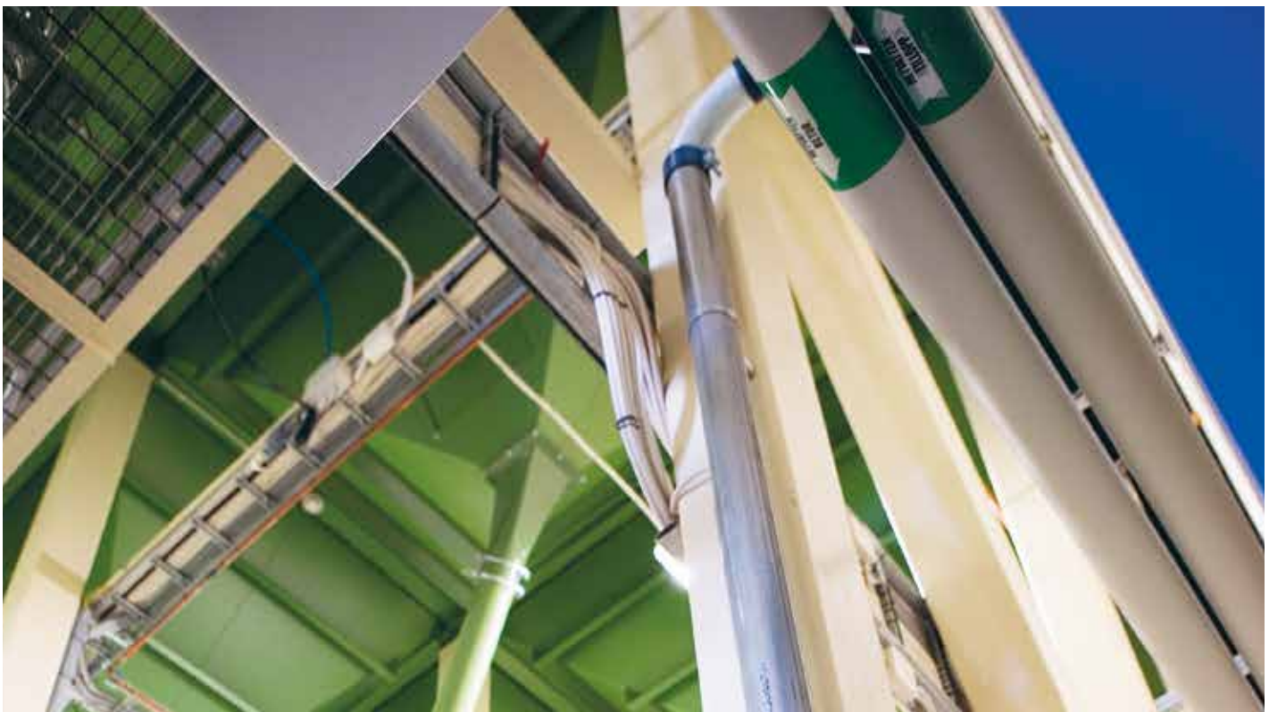
Dustcontrol Steel Tubing System
