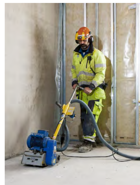
Suction is available on each floor.
